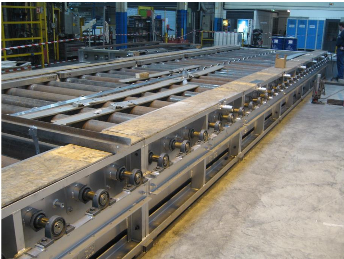
Installation supervision – Check the installation of the furnace heat treatment at SJI St Jean d’Ardières (France)
