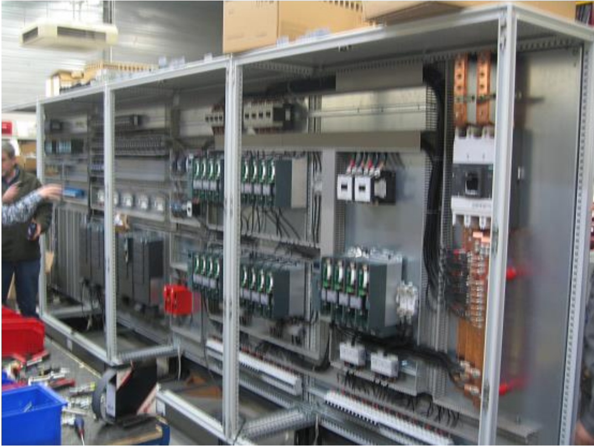
Manufacturing inspection – Check of the electrical cabinets at Stemi St Denis en Bourg (France)
