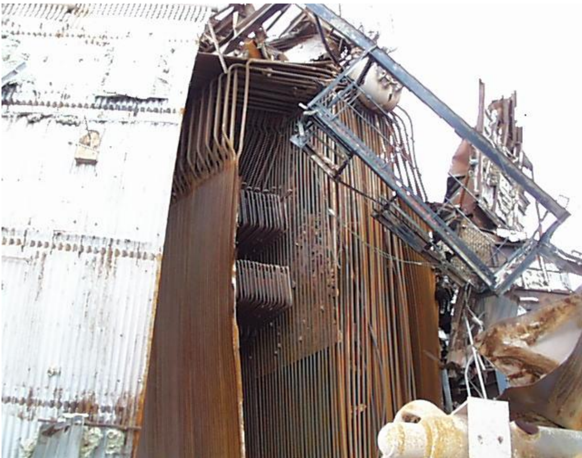
Industrial damage expertise – Site of Sonatrach at Skikda (Algeria) Damage on the Clark Chapman boiler
