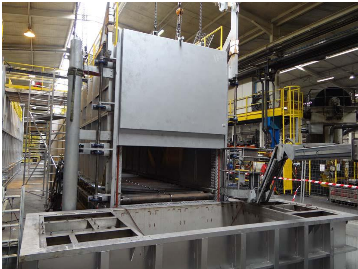
Erection supervision - Normalization furnace with quench tank for Aluminium parts at (Saint Jean Ind. France)
