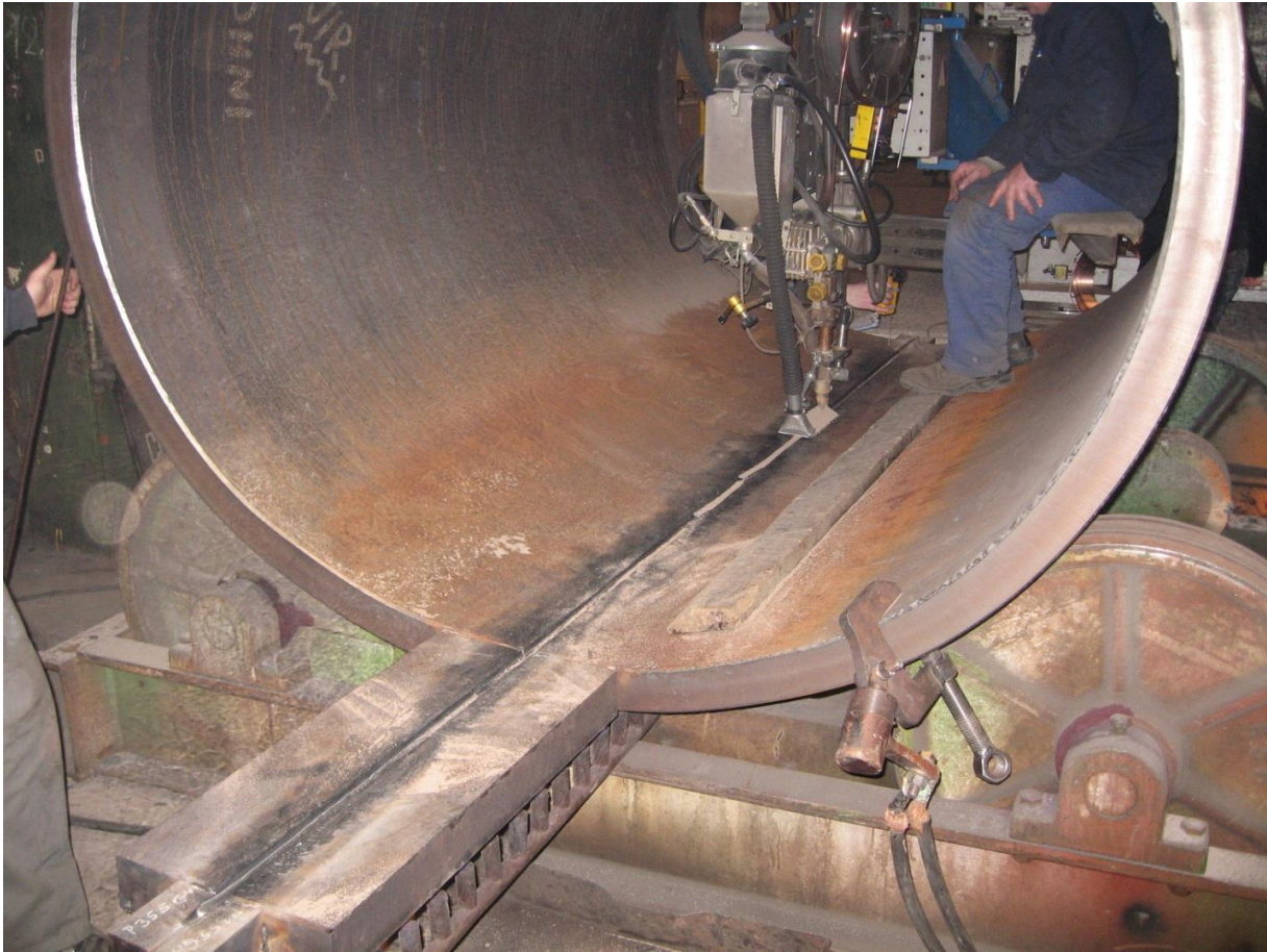
Manufacturing supervision - Condensate tanks for Flamanville (FR) at Excon Radek Kralove (Czech Republic)
