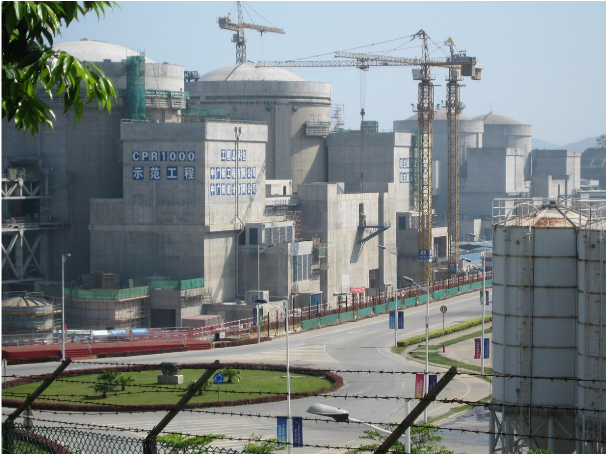
Site supervision - On site Moisture Separator Reheater (MSR) installation supervision at Ling Ao (China)
