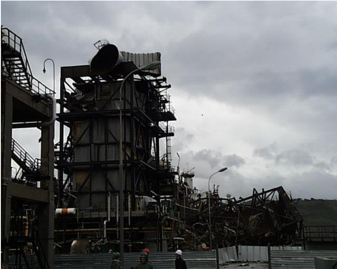
Industrial damage expertise – Site of Sonatrach at Skikda (Algeria) Damage on the Alstom boiler
