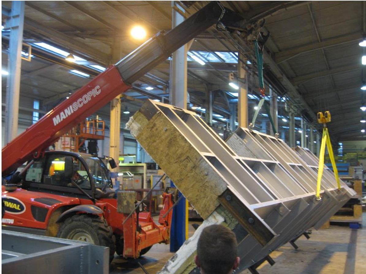
Installation supervision – Check installation of the T6 unit at SJI St Jean d’Ardières (France)
